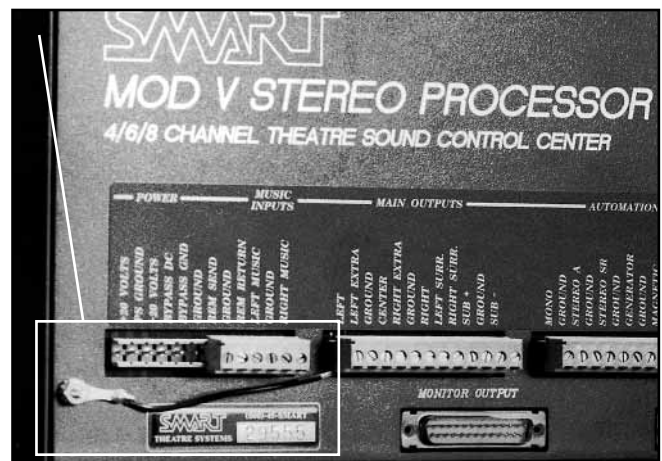
Rear view of MOD V showing the special ground wire.
